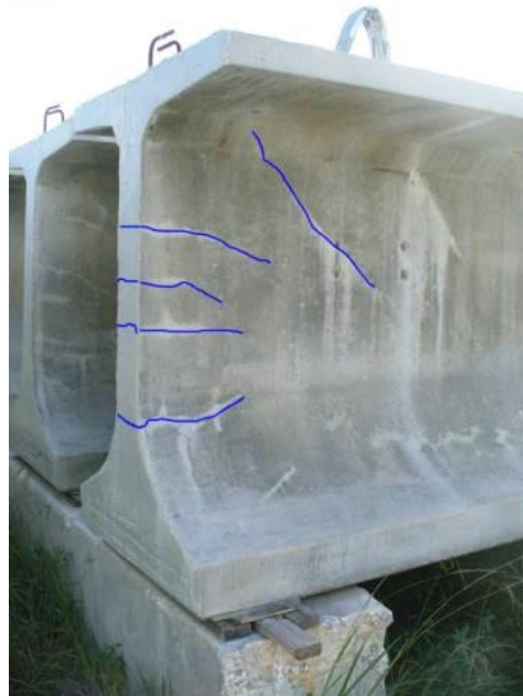
Figure 1. End-region web-splitting cracks enhanced in blue 2
