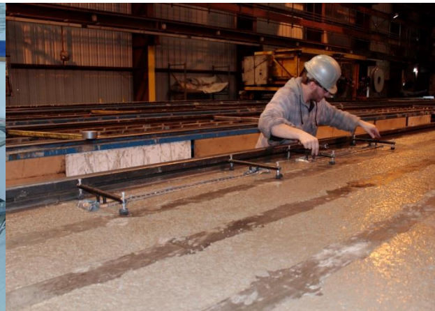
(b) Placing steel bar with brass inserts on the concrete cast surface
