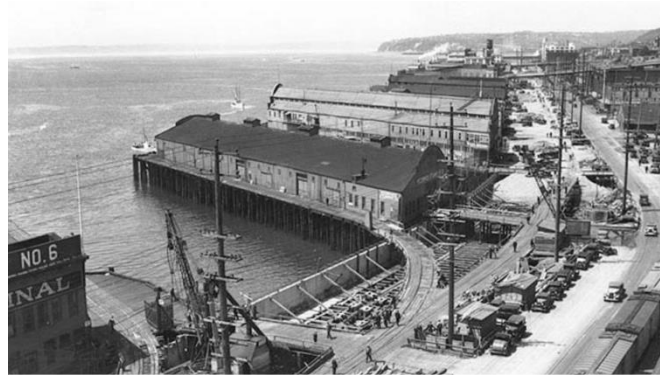
Railroad Avenue and Original Seawall Under Construction Showing Precast Wall Panels (historical photo from waterfrontseattle.org)
