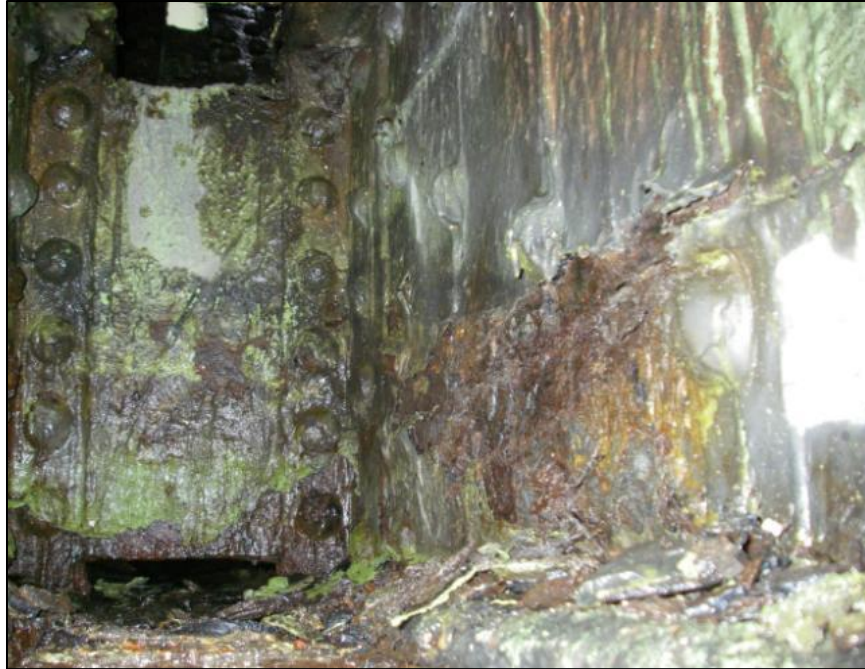
Fig. 2 Typical Deteriorated Steel Gusset Plate Connection
