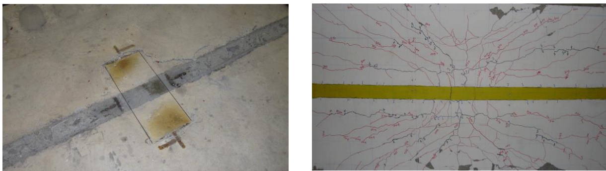
a) Slab top surface at wheel load location
