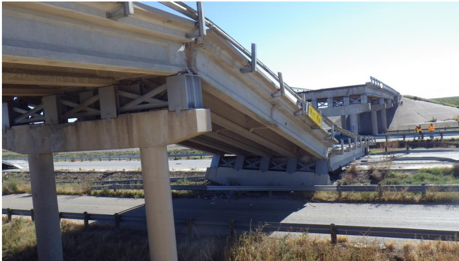
Figure 13 Overview of Damaged Bridge – IH 20 Underpass at FM 2599
