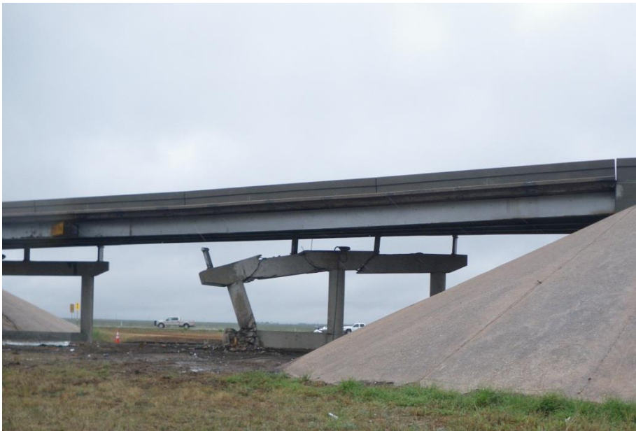
Figure 1 Overview of Damaged Bridge at US 84 over IH 20 in Nolan county
