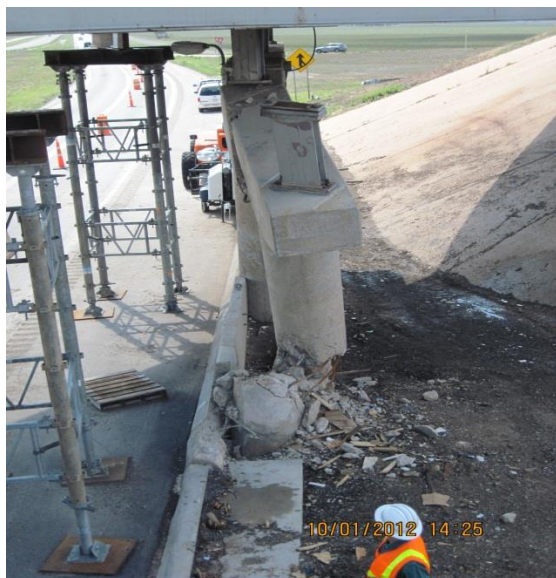
Figure 15 Damaged Columns Struck by 18-wheeler truck
