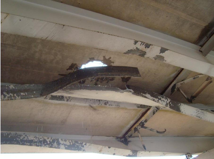
Figure 8 Damaged Bridge Concrete Deck
