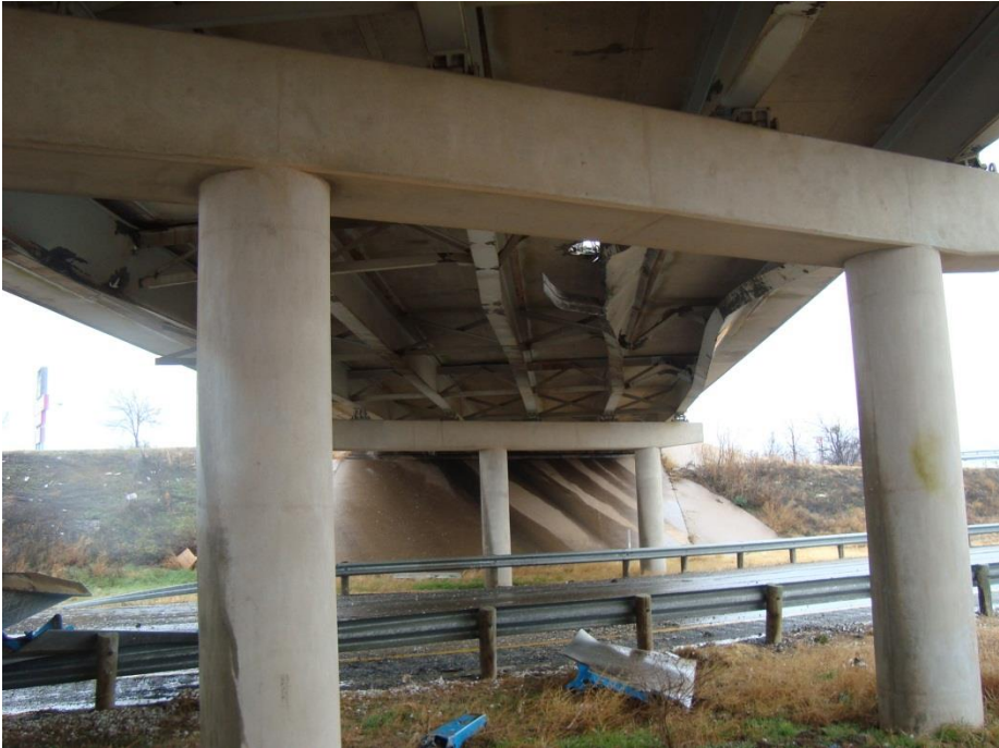
Figure 9 Damaged Bridge (Under view)
