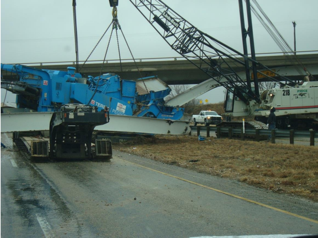
Figure 6 Damaged Bridge – US 180 Overpass at US 84 in Snyder County
