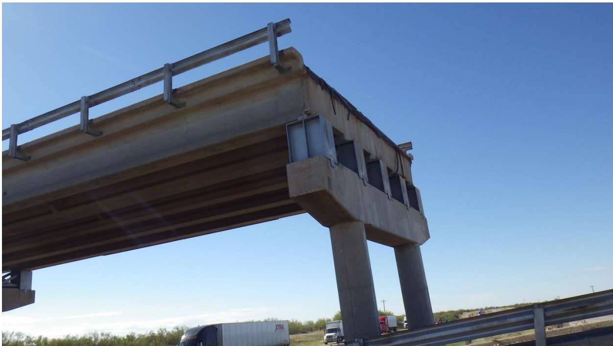
Figure 14 Partial Collapse of Columns of Interior Bent
