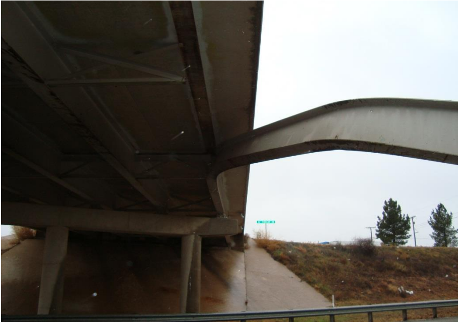
Figure 7 Steel Girder Damaged by the 18 Wheeler Truck
