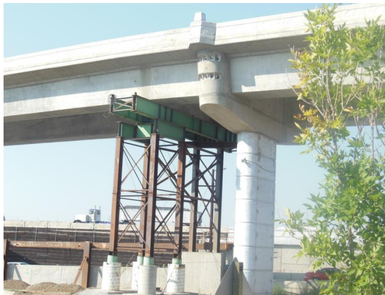
Figure 9: Example of Falsework Tower
