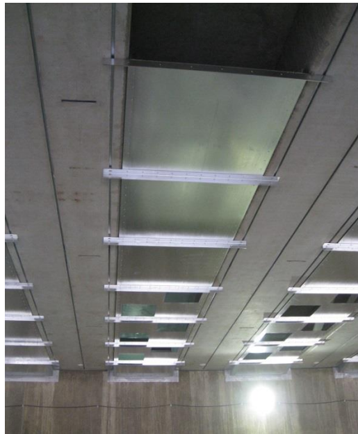
Figure 21: Unistrut inserts on box girders, formed ventilation ducts can be seen between girders.
