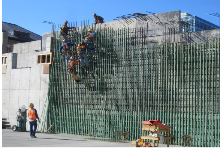
Figure 12: Cast in place wall construction, exterior wall shown with forms in the back-ground.
