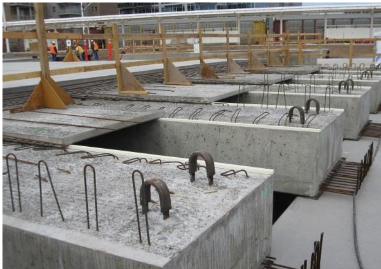
Figure 25: Construction Cross section showing precast panels on Box Girders, with a portion of cast deck beyond.
