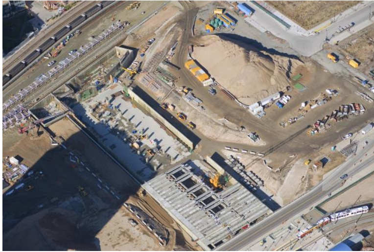
Figure 8: First stage construction. North is to the top right, the new LRT station is to the upper left and the existing LRT station is at the bottom right.
