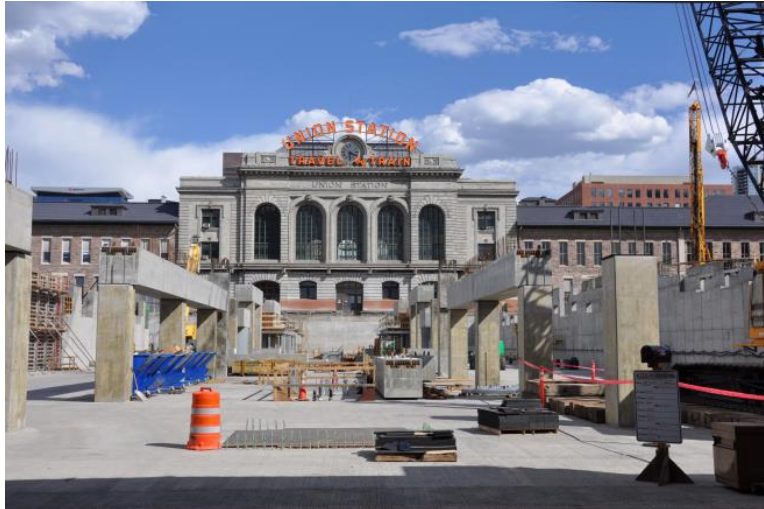
Figure 18: Bent cap erection staging, DUS can be seen in the background (Looking East).
