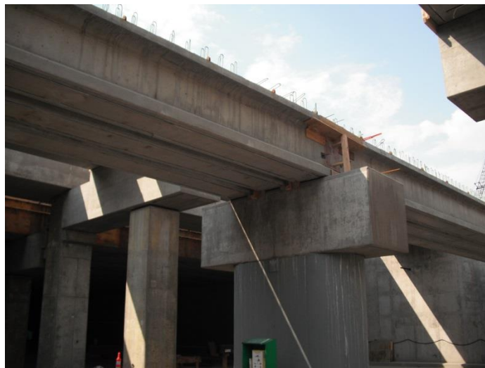
Figure 26: CRT train bridge for a single track, with clipped BT girder in place.
