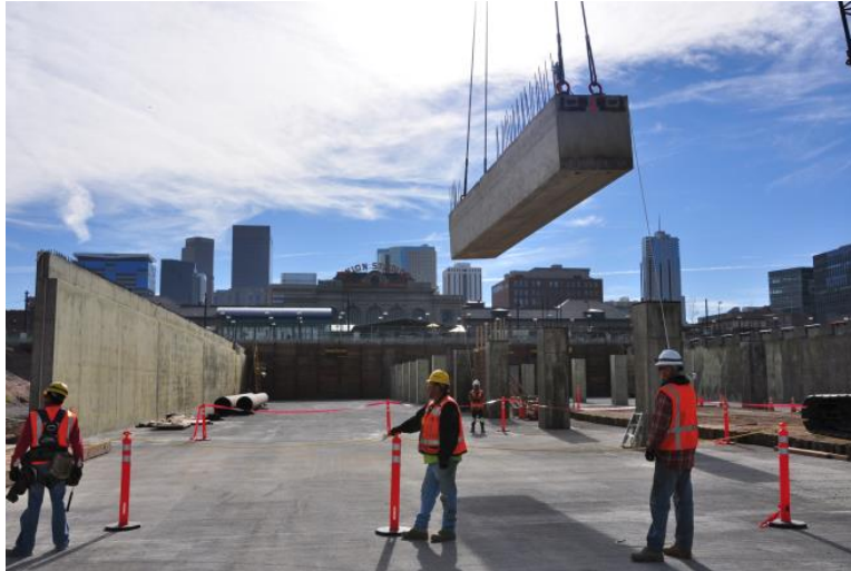
Figure 16: Erection of the first precast bent cap, looking east the historic DUS and Denver skyline in the back ground.
