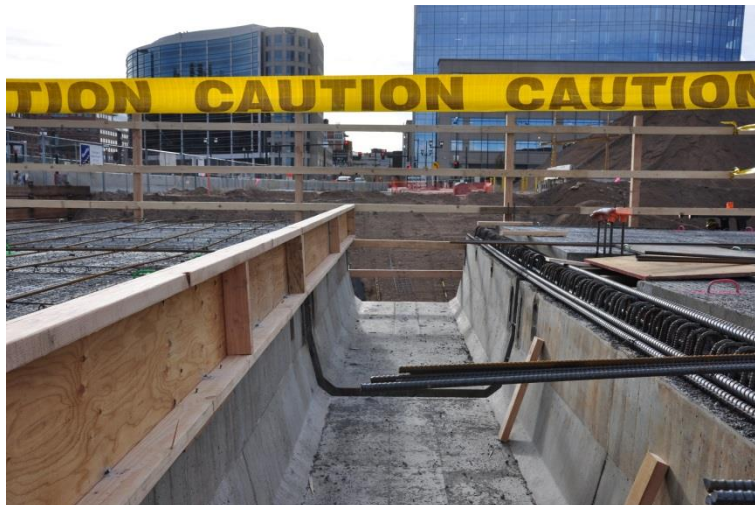
Figure 23: Tub Girder utility trench with deck formwork to the left and right.
