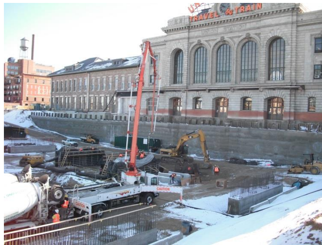
Figure 9: DUS shoring wall in the background, Rail bridge foundation construction in the foreground.
