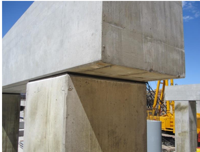
Figure 15: In place precast bent cap at the CRT platforms, final placement shown on cast-in-place columns.
