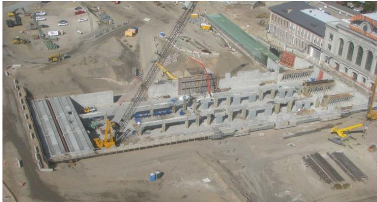
Figure 10: Second stage construction, North is to the Top Left, the historic station can be seen to the right.
