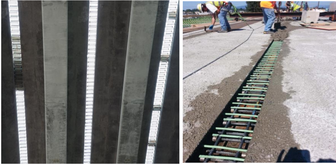
Figure 3: View Underneath Decked-Bulb Tee Girder Connection (Left) Casting of the Deck Closure between Girder Flanges to provide a Full Flexural-Shear Connection (Right)
