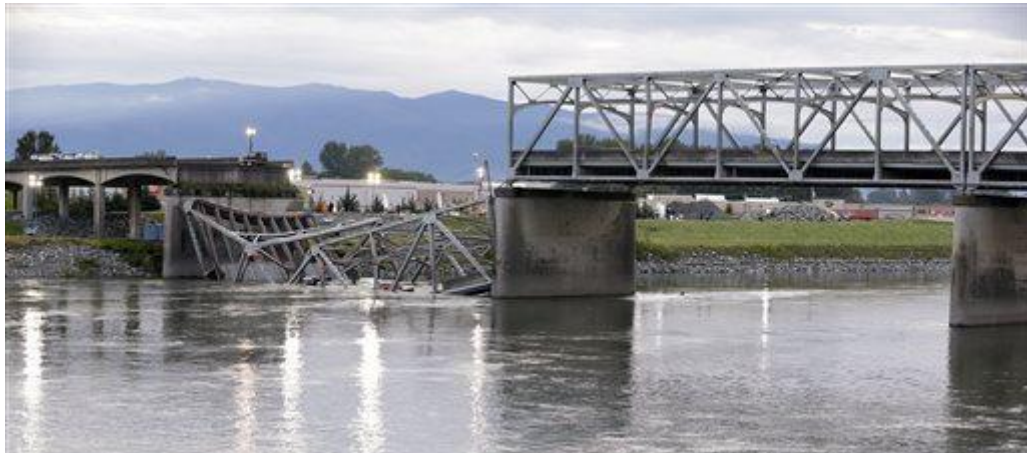
Figure 1: View from the South Bank of the Skagit River Bridge Collapse
