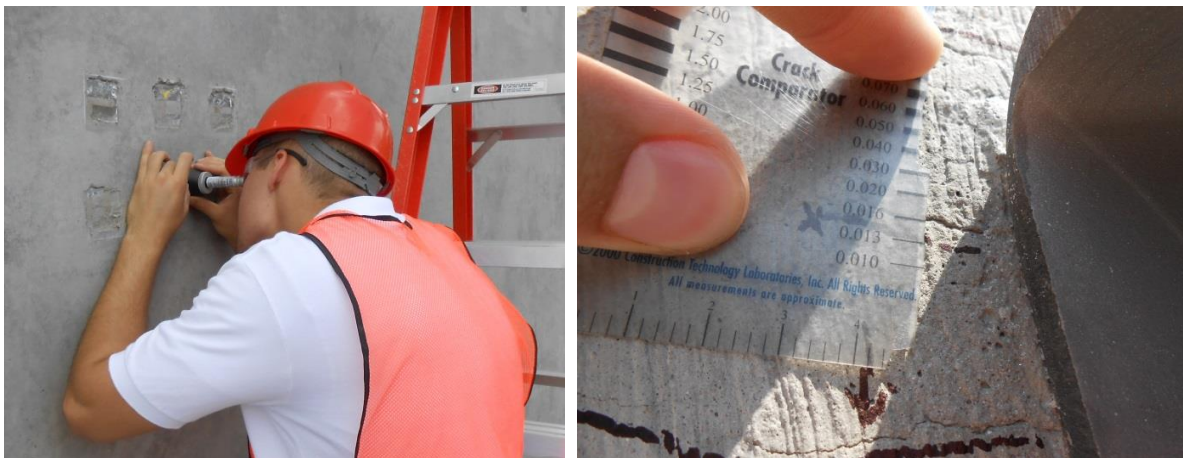
302 303 Figure 6 - Measuring crack with microscope (left) and card (right)
