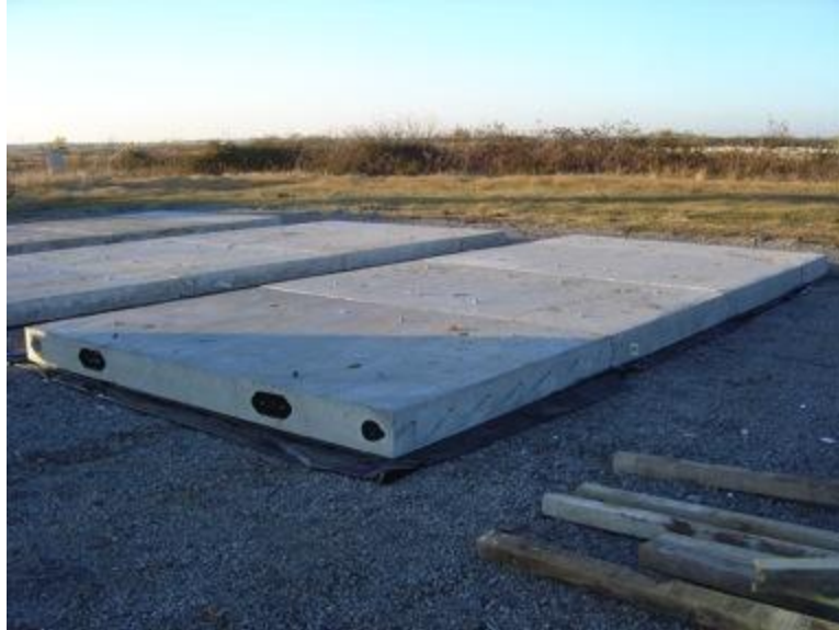
Figure 9 Precast Pavement Panels are assembled and readied for Post-Tensioning. The Test Panel in the foreground is Test Panel III which is 10 in. thick. It features longitudinal and transverse prestressing of approximately 240 psi. The visible ductwork in Test Panel III is fitted for two two-strand tendons and two-four strand tendons.
