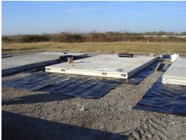
Figure 8 Precast Pavement Panels are assembled to form the Test Pavements I, II and III.
