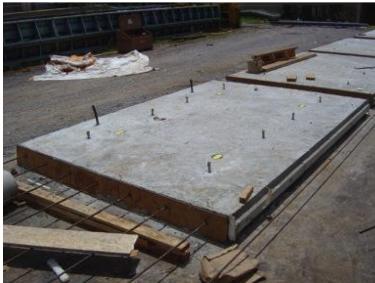
Figure 5 Completed panel. The shear key is visible in the panel, as are the grouting ports for grouting the under-slab voids.
