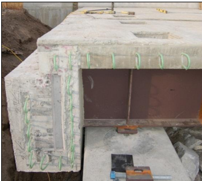
Figure 5: Overhanging backwall at abutment
