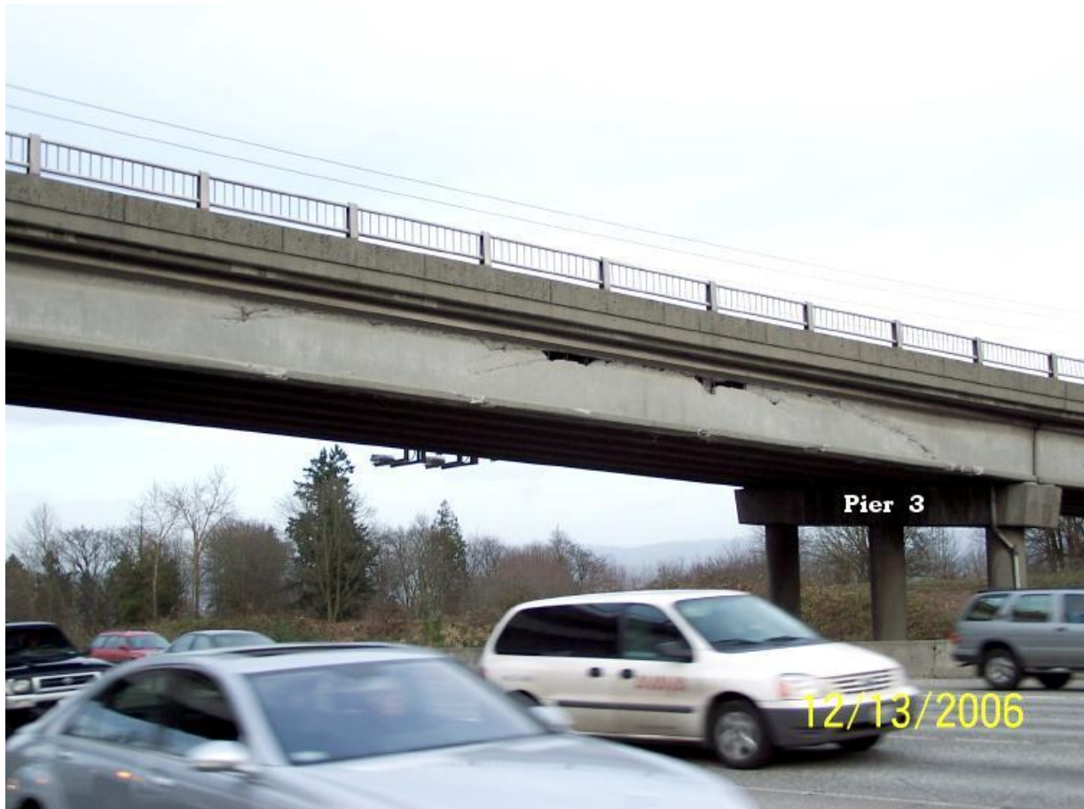
Figure 10 Damage to the South 178 th Street Bridge
