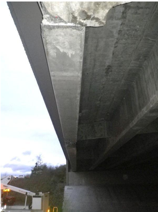
Figure 14 Lateral displacement of girder at center pier diaphragm
