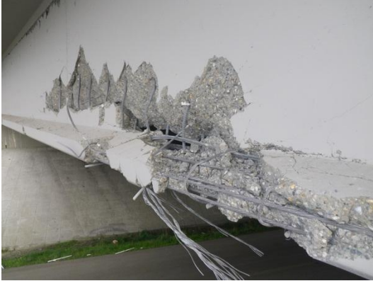
Figure 13 Olympic Road Bridge girder damage at point of impact
