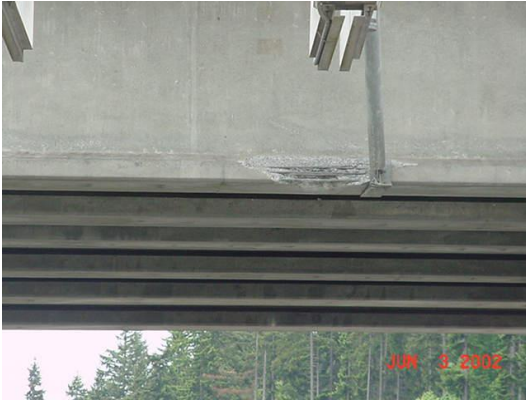
Figure 2 Impact site and damage to the Trigger Avenue structure
