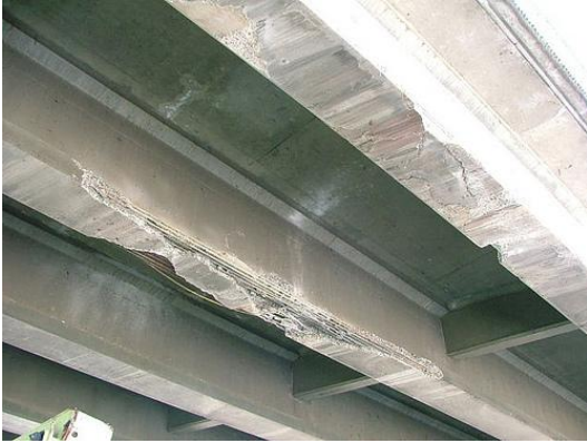
Figure 8 Damage to second and third girders
