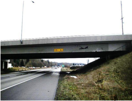
Figure 15 Impact damage to the 24 th Street Bridge
