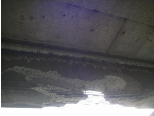
Figure 11 Girder damage on the 113 th Avenue Bridge
