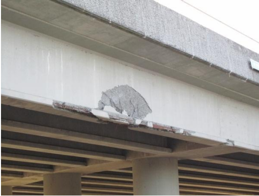
Figure 12 Olympic Road Bridge Girder Damage
