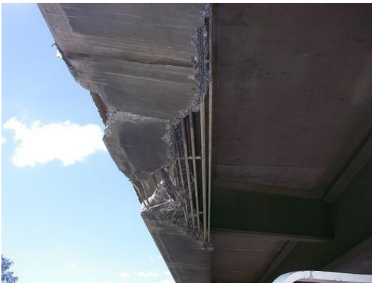
Figure 7 Damage to girder receiving direct impact
