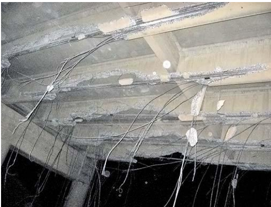
Figure 6 Damage to the Easton Road Bridge
