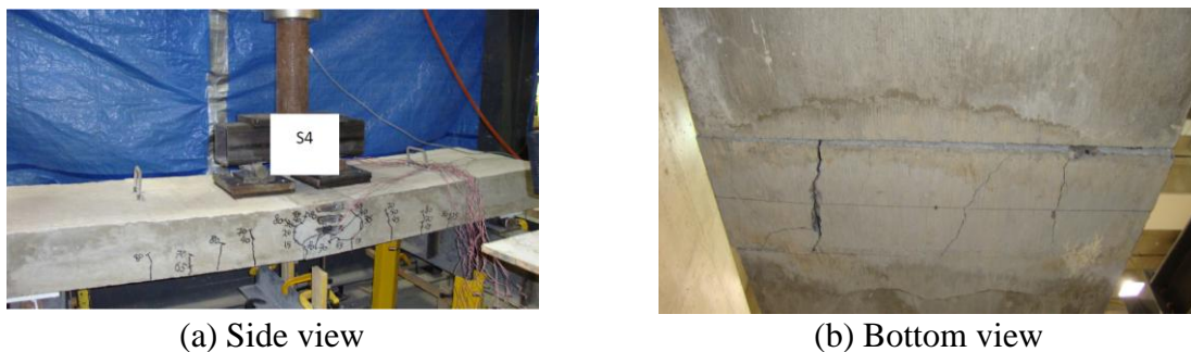
Fig. 11 Crack behavior for deck slab S4
