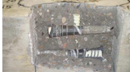
(b) Bar head breakage in slab S4
