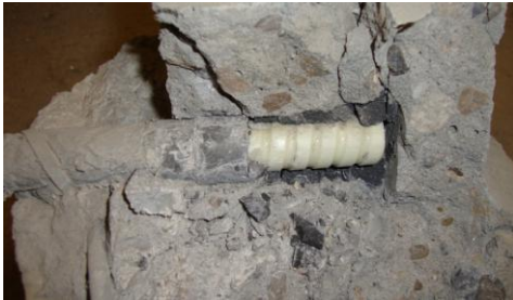
(c) Bar head breakage in slab S5
