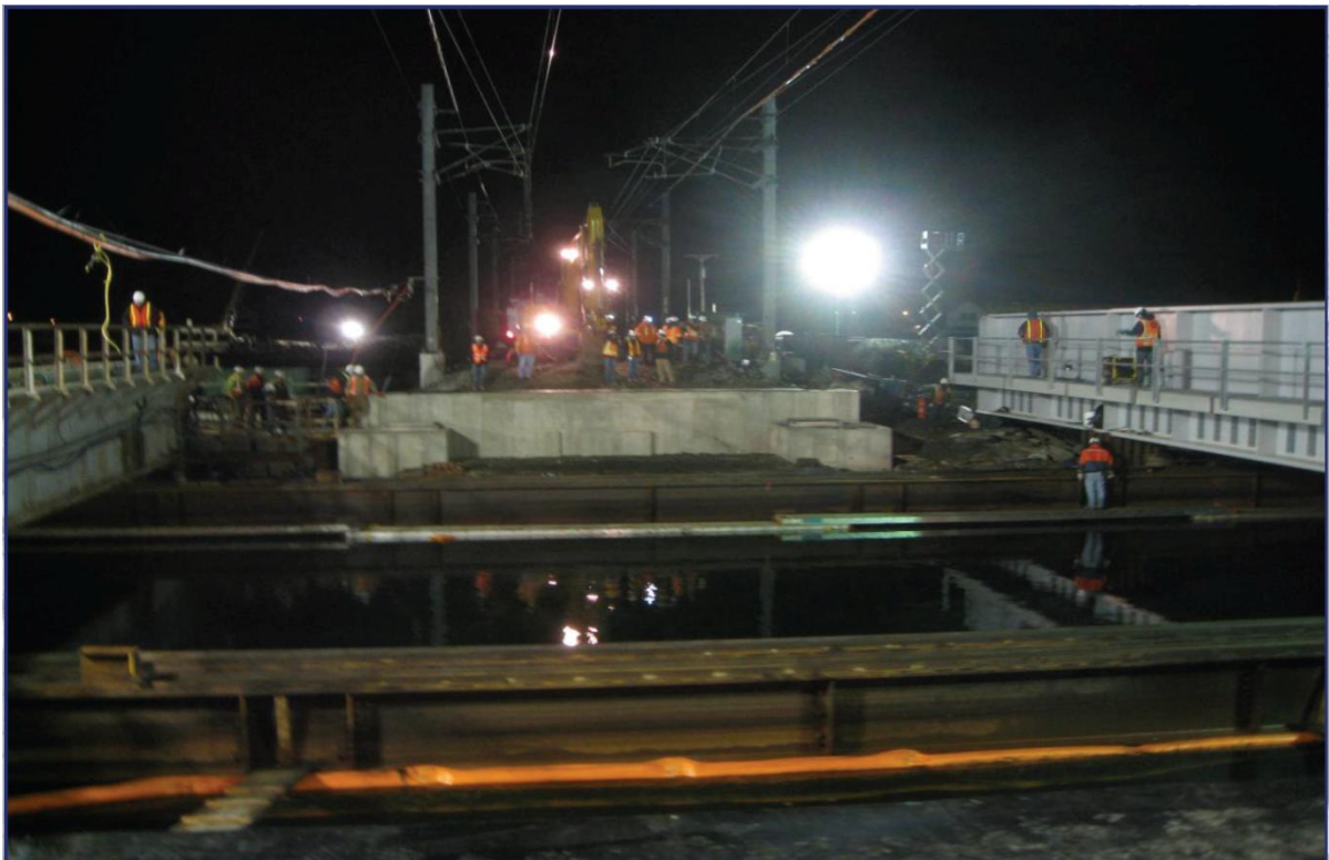
Fig. 8 Existing Bridge Rolled Out and New Bridge to Be Rolled In (AREMA)
