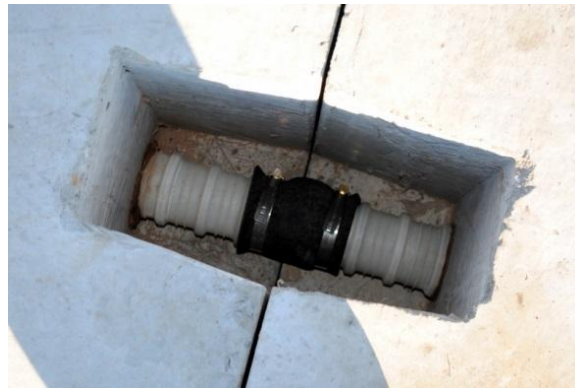
Figure 4 – Post-tensioning duct coupler in handhole between mat foundation segments
