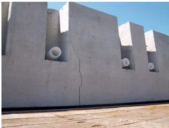
(a) Cracked mat foundation segment
