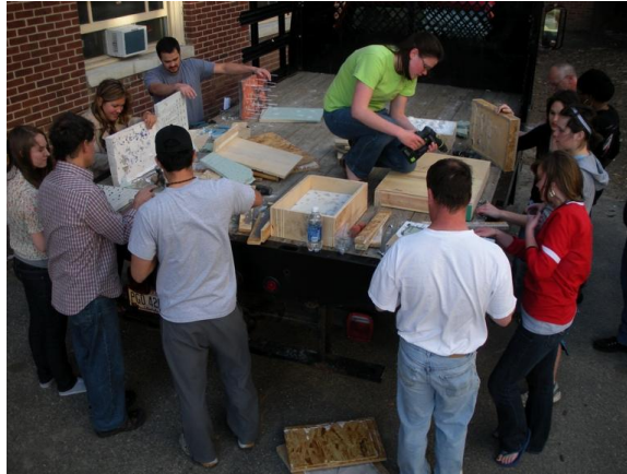
Fig. 6 “Stripping Party” at University working from precast company’s flat bed truck which is strategically parked close to the dumpster.
