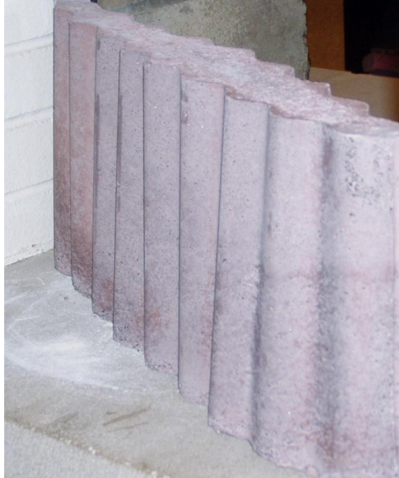
Fig. 26 Corrugated metal formed the sides of the formwork clamped together at the ends only. The mass of the uncured concrete created the intended entasis at the center.
