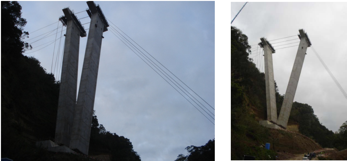
Fig. 10. System of stays arranged in the opening of the first pair of piers
