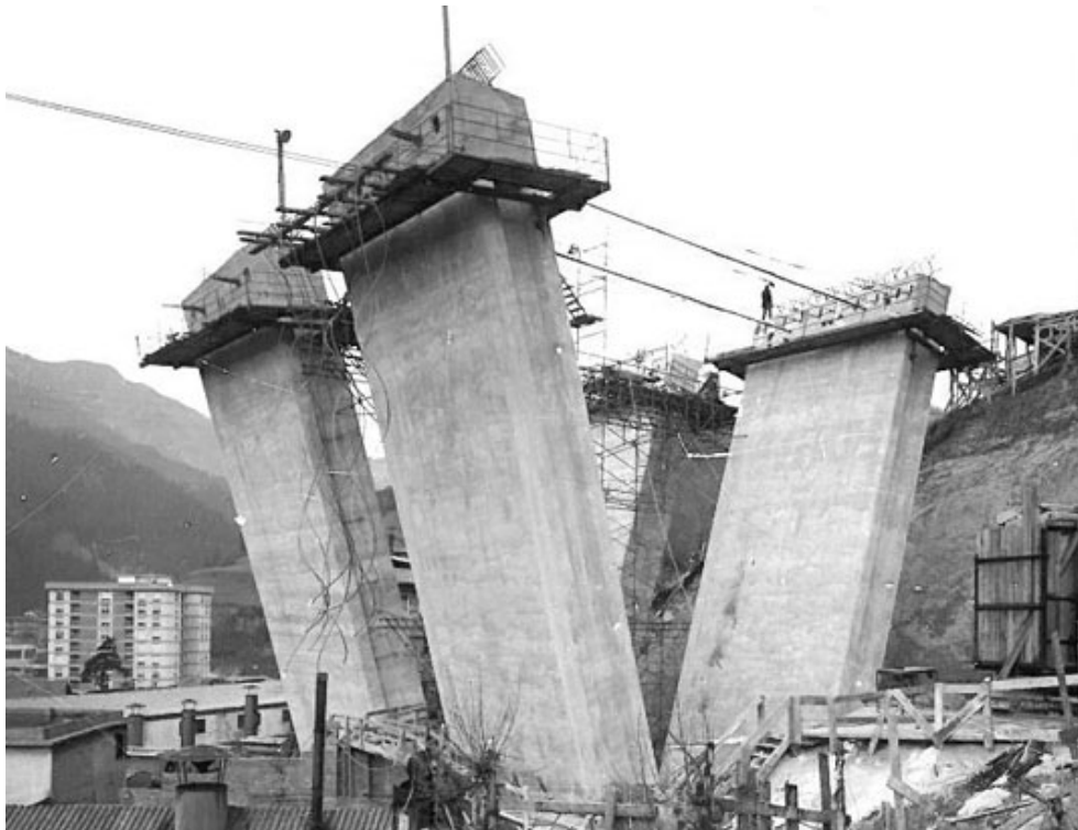
Fig. 2. Rotation of Chonta viaduct piers. Opened in 1973
