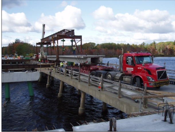
Fig. 20 Gantry crane and rail system
