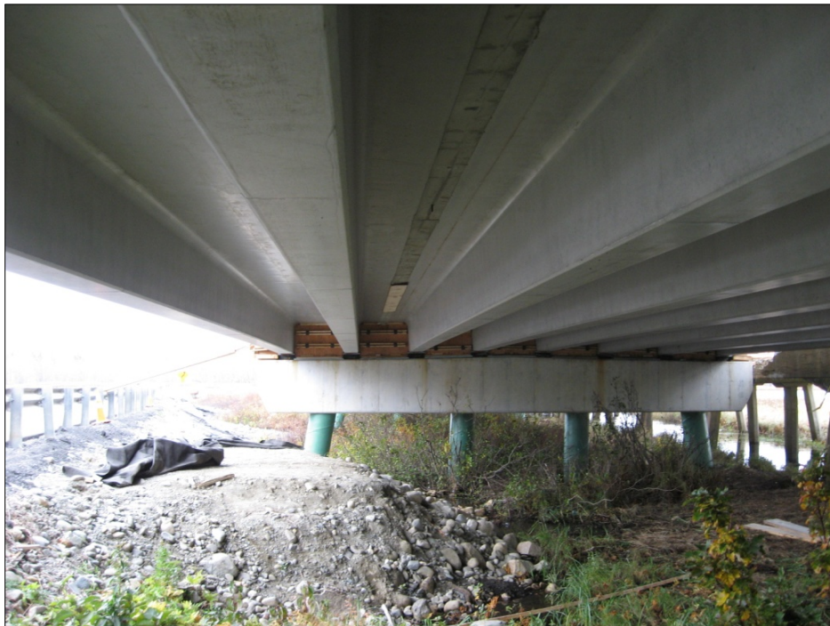
Fig. 8 Underside of NEXT D beam span between temporary detour road and existing bridge
