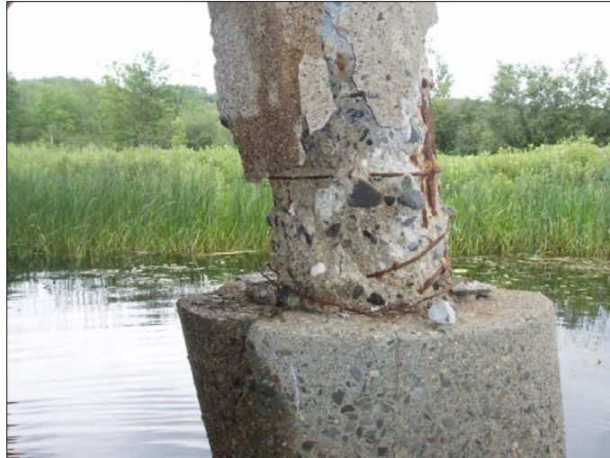
Fig. 18 Existing concrete pile requiring repair
