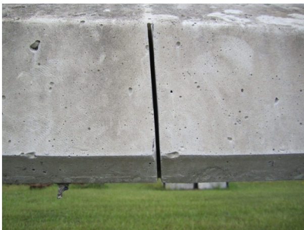
Fig. 23: Damaged full scale PSC beam
