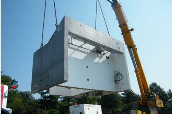
Figure 24: The monolithic center core, the “brains” of the house, which contains all of the mechanical, electrical, and plumbing systems also supports the inverted-hip roof being craned into place during the Washington, DC build, September 2011.
