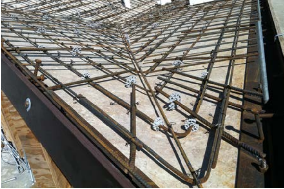
Figure 22: “the boat” being formed within the plywood jig specially fabricated for its manufacture. Note the amount of steel reinforcing to withstand the roof cantilevers.
