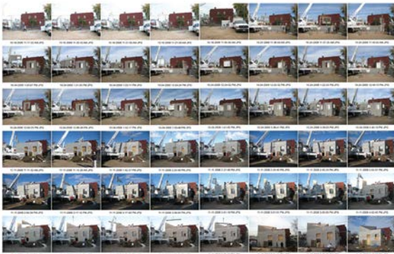
Figure 10: A portion of time elapsed photography of the 3-day erection of PREttyFAB's shell.
