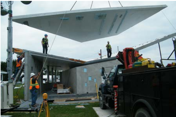
Figure 25: Large insulated sandwich roof panels being craned into place during the Washington DC build, September 2011. Note the exposed layer of graphite impregnated expanded polystyrene of the set panel on the left.
