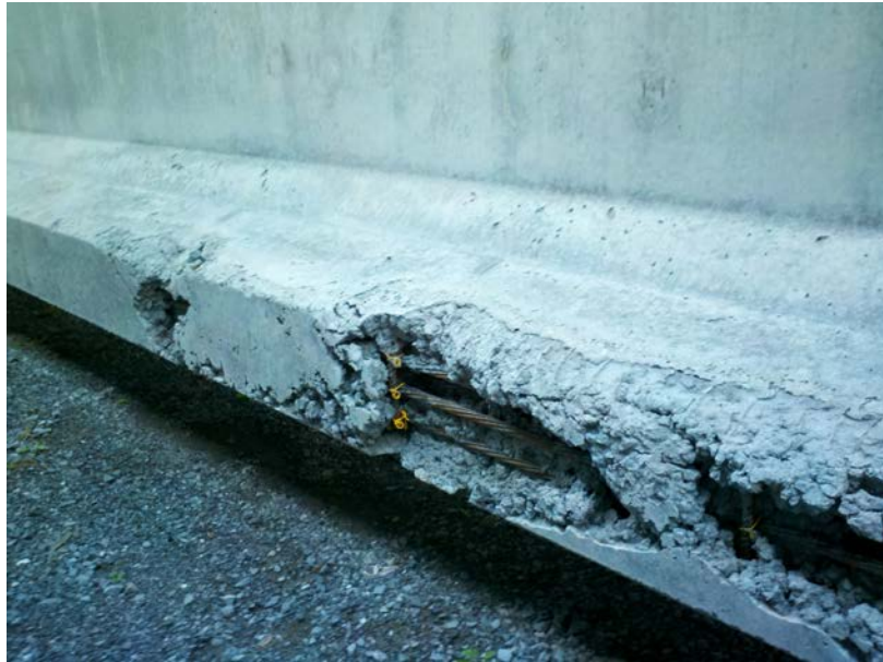
Fig. 5 Rejected Bridge Girder with Consolidation Voids
