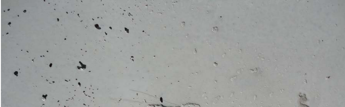
Fig. 2 Partially patched surface of a structural element
