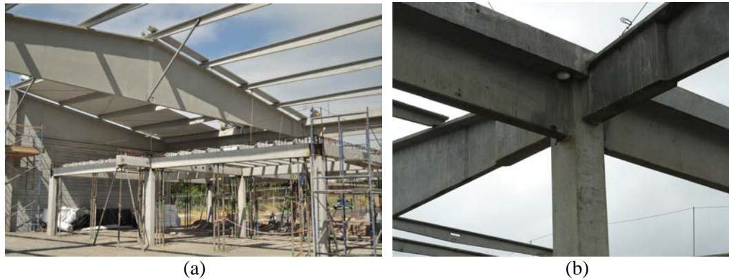
Fig. 2. Precast Industrial Building in Costa Rica. a) Main span b) Roof beam-column wet connection
