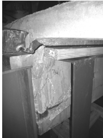
Fig. 7 Shear Failure of the Beam
