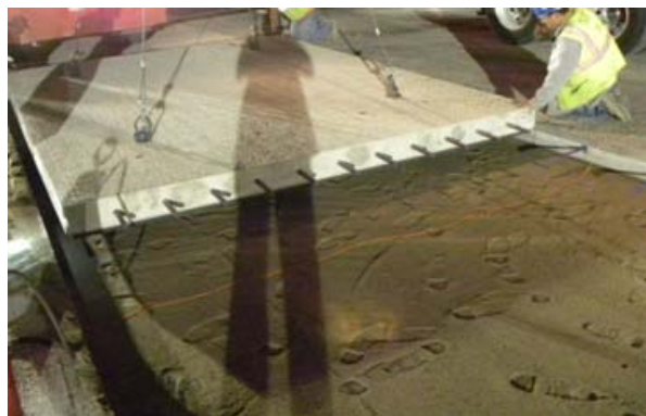
Fig. 13 Poorly Compacted Fine-grained Bedding Layer
