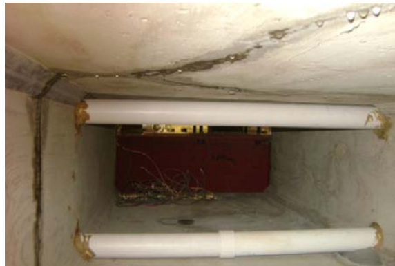
Fig. 17 Interior View of Cracking at Flange along North-East Side of Joint
