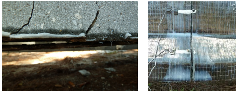
Fig. 12: (left) Debonding of soffit CFRP; (right) Rupture of longitudinal & transverse CFRP
