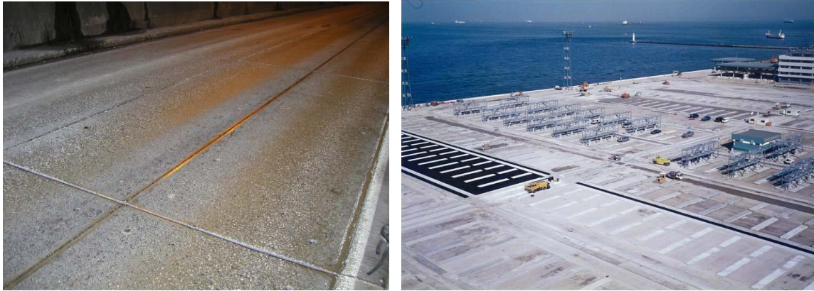
Fig. 10 Typical Tunnel and Port Applications
