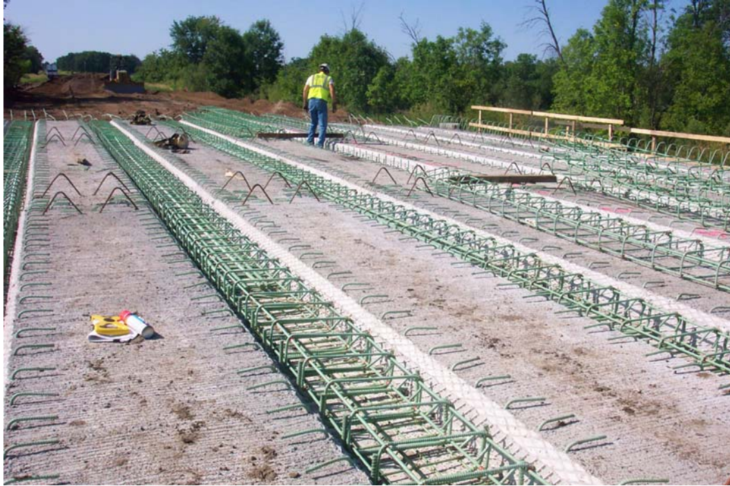
Fig. 2: Photograph of PCSSS construction showing inverted-tee precast beams and drop-in cage reinforcement prior to CIP placement
