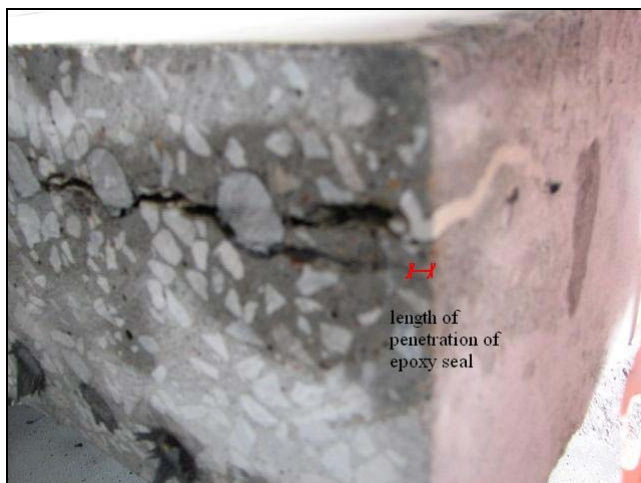
Figure 3. End zone cracking extends vertically and horizontally (Girder 1)
