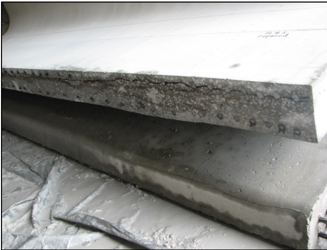
Figure 2. End zone cracking extending the full length of the web (Girder 1)
