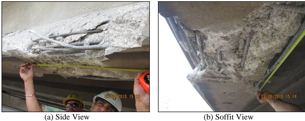
Fig. 5: Girder #1 Impact Damage
