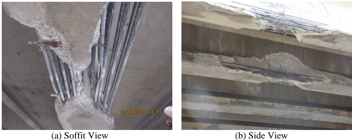
Fig. 6: Girder #4 Impact Damage
