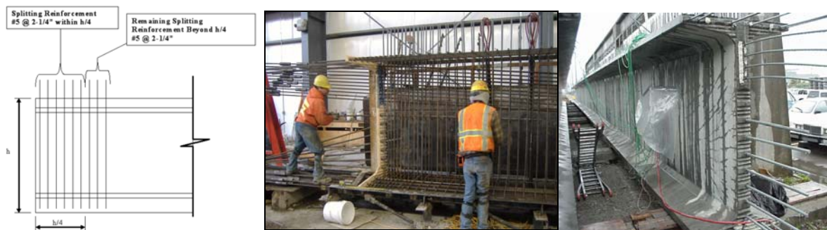
Fig. 6: Splitting Reinforcement at Girder End Zone
