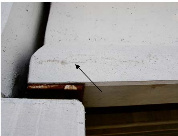
Fig. 3 Longitudinal End Zone Cracking Due to Anchorage Stresses
