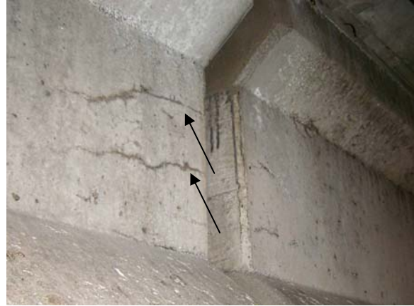
Fig. 2 End Zone Cracking in Interior Beam
