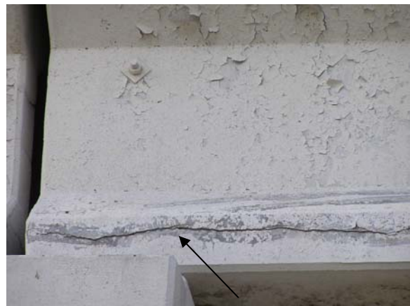
Fig. 4 Longitudinal End Zone Cracking Due to ASR/DEF
