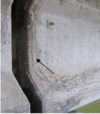
Fig. 5 Cracking in Beam Web Due to ASR/DEF
