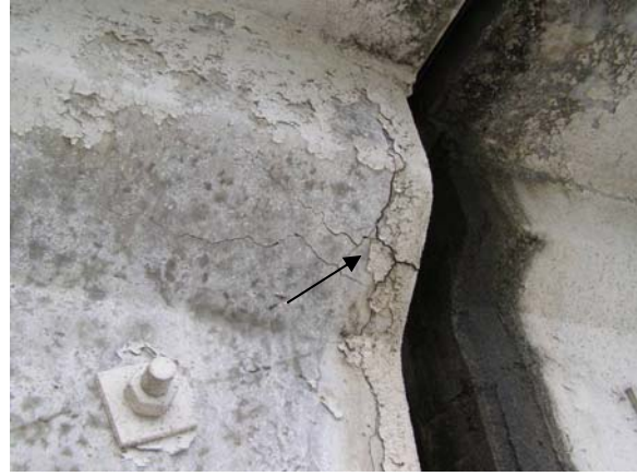
Fig. 6 Cracking in Beam Top Flange Due to ASR/DEF
