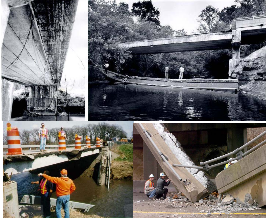
Figure 3: Adjacent non-composite box beam failures (from top left clockwise: Ohio bridge pre-failure, Ohio bridge post-failure, Pennsylvania failure, Illinois failure)
