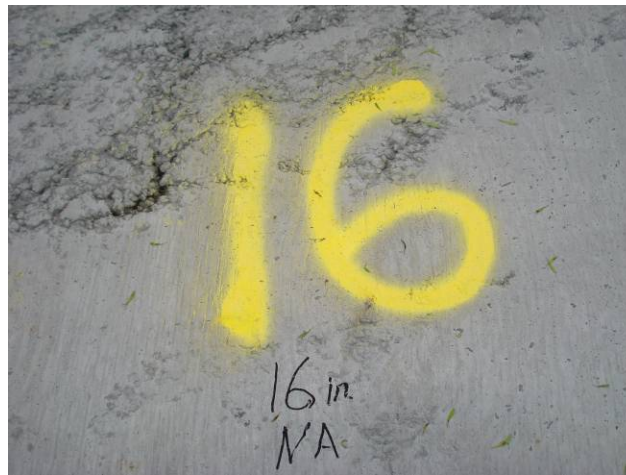
Figure 2. Wall 16 Showing Poor Slump Flow
