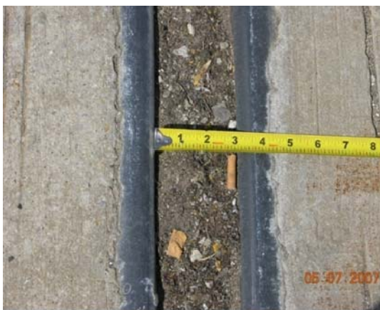
Joint Filled with Debris
