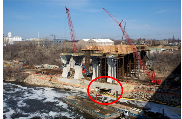
Figure 5 – Footing Straddling Storm Drain
