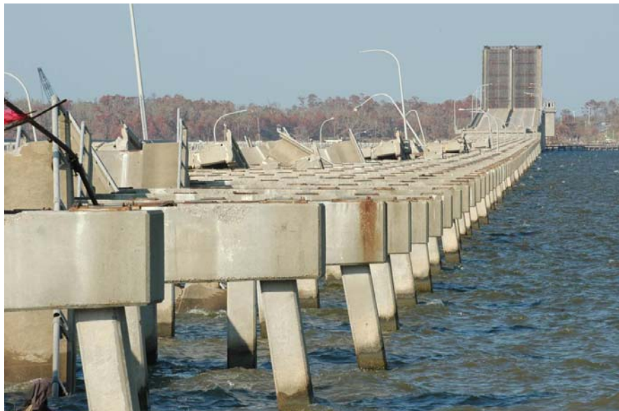
Fig. 1 Storm Damaged Bridge
