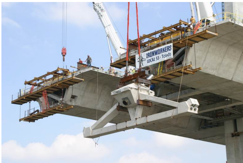
Fig. 7 Precast delta frame is lifted into place using a crane on the cantilever tip.
