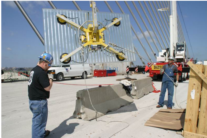
Fig. 21 A partially mirrored glass panel is prepared for installation into the upper pylon.
