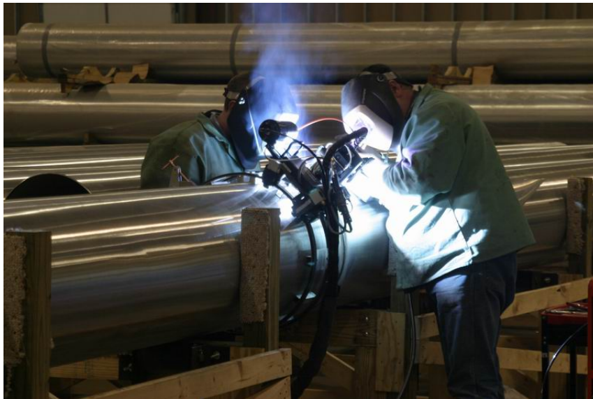
Fig. 15 An orbital welding machine is used to weld stainless steel sheathing sections.
