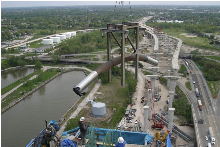
Fig. 14 A stay cradle and its support frame is set into the pylon formwork by the tower crane.
