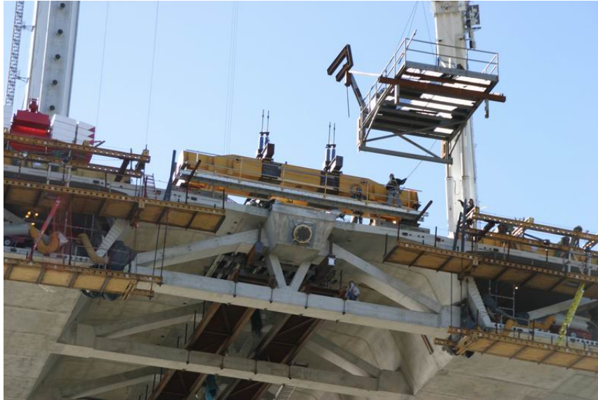
Fig. 10 Stay stressing platform being lifted into place at the end of the main cantilever.
