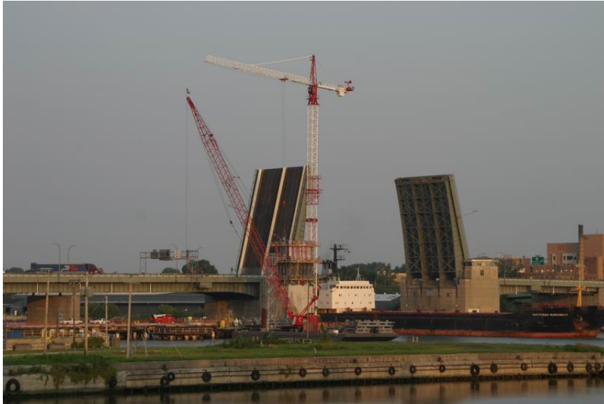
Fig. 1 The Craig Memorial Bridge opens to allow passage of a Great Lakes freighter.
