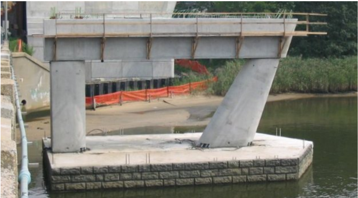
Fig. 13. The precast columns and cap beam have been erected to complete the first pier. The cap beam will be prepared for cast-in-place concrete leveling pads.
