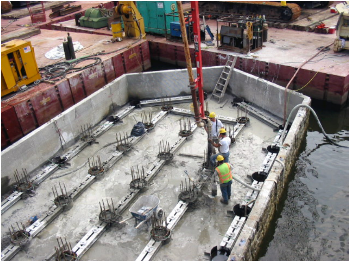
Fig. 10. Work being performed inside a cofferdam. Structural support of the cofferdam has been transferred to the pile heads. Piles are being filled with concrete.
