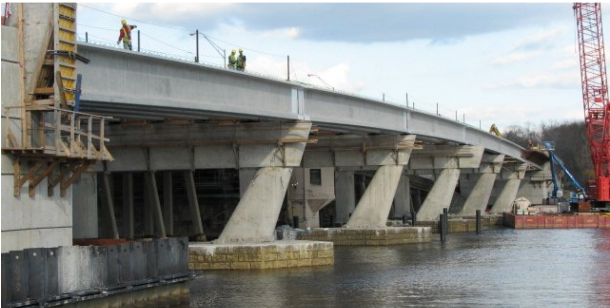
Fig. 17. Eastbound bridge piers 1 through 5 have been completed, and the bulb tee girders have been erected.
