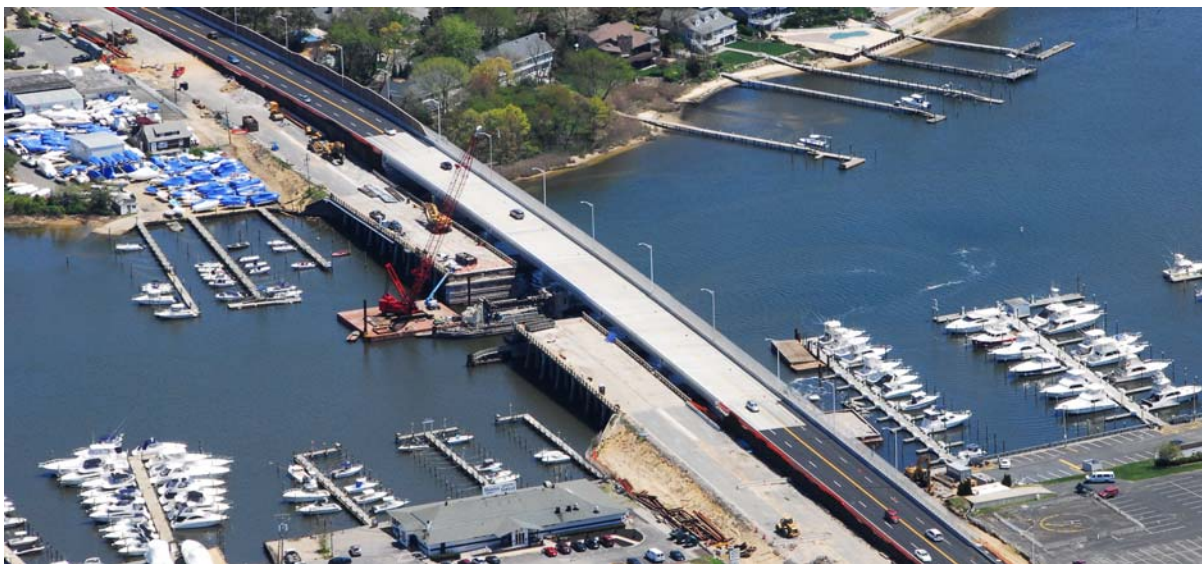
Fig. 4. Traffic has been shifted onto the newly completed eastbound half of the bridge and the existing bridge is being demolished.
