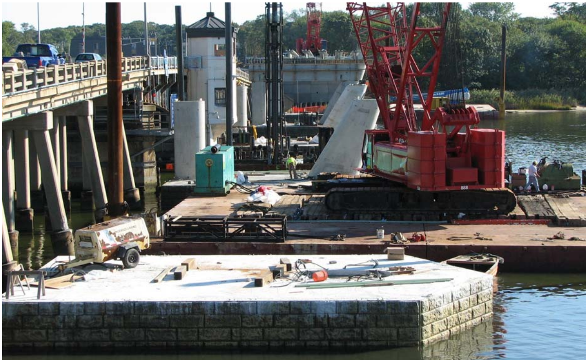
Fig. 15. Crews work on multiple piers at the same time. Piers are shown in various stages of completion.
