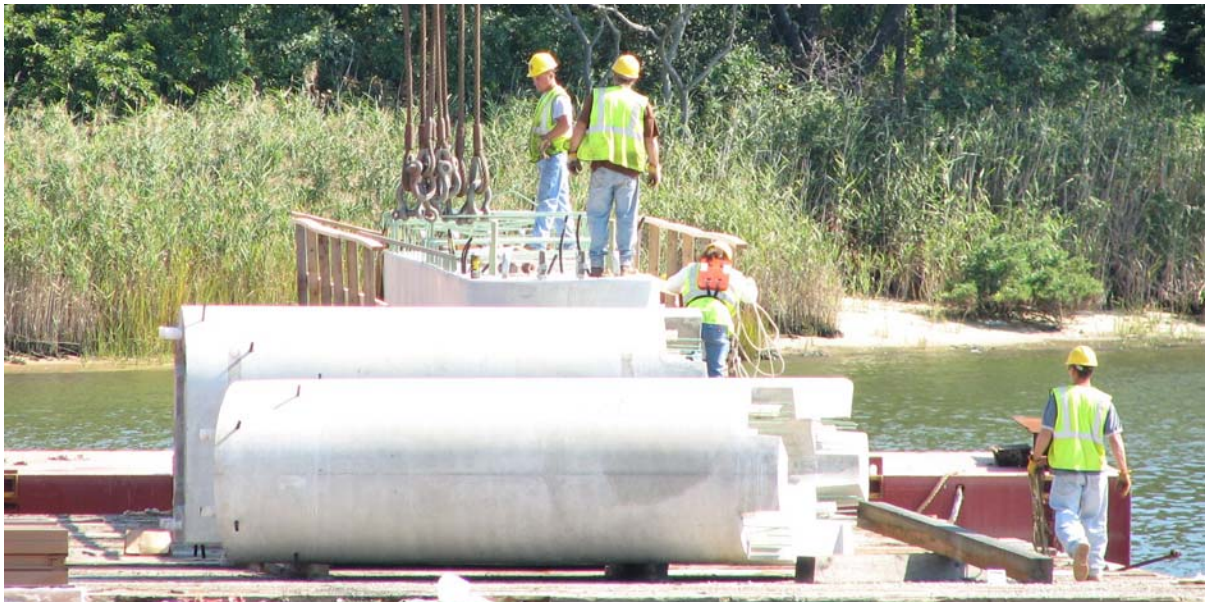
Fig. 11. Precast pier columns and a cap beam have been loaded on a barge and are being prepared for erection.
