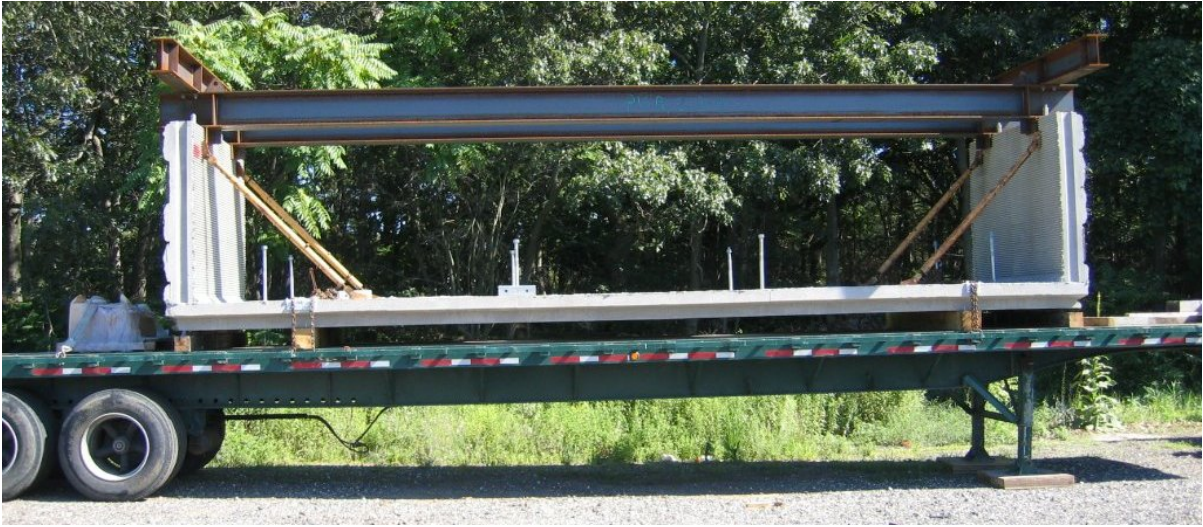
Fig. 8. Cofferdam section has been trucked to the project site and fitted with lifting beams.
