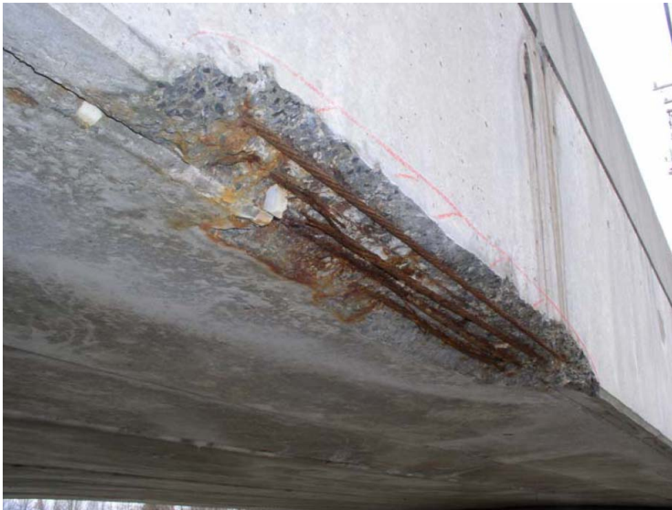
Figure 11 - Typical Impact Damage
