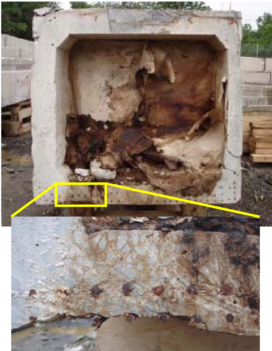
Figure 5 - Cross Sectional Slice of Test Beam 1
