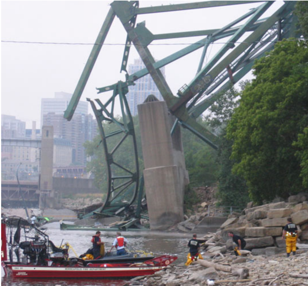
Fig. 2 Failure of a Complete Bridge
