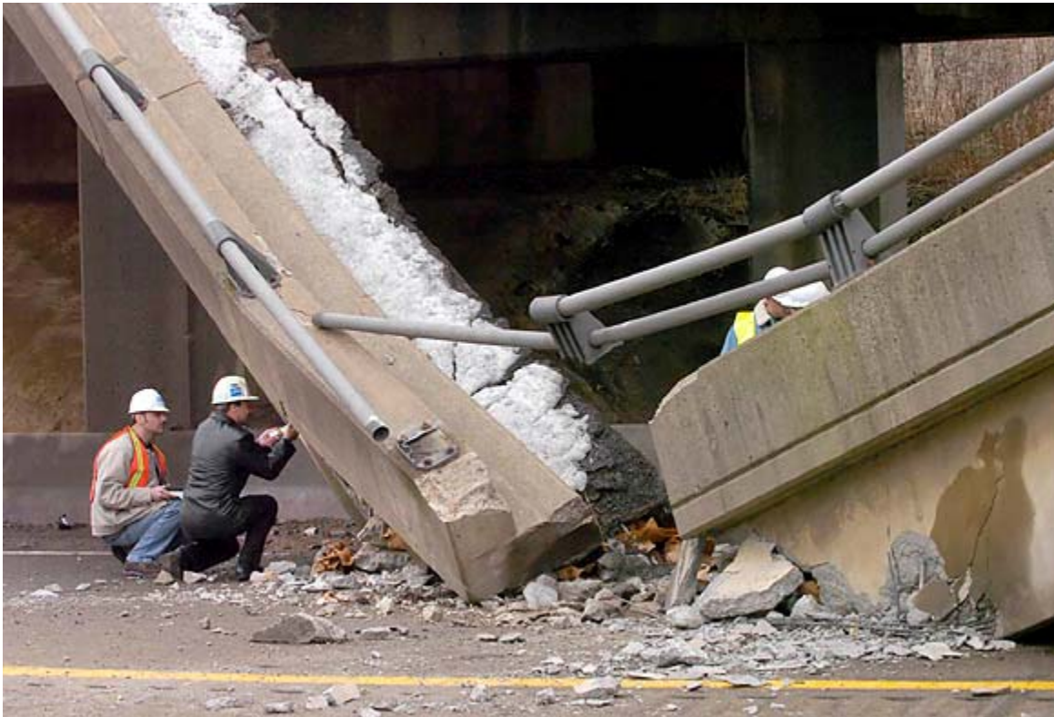
Fig. 1 Failure of a Bridge Component
