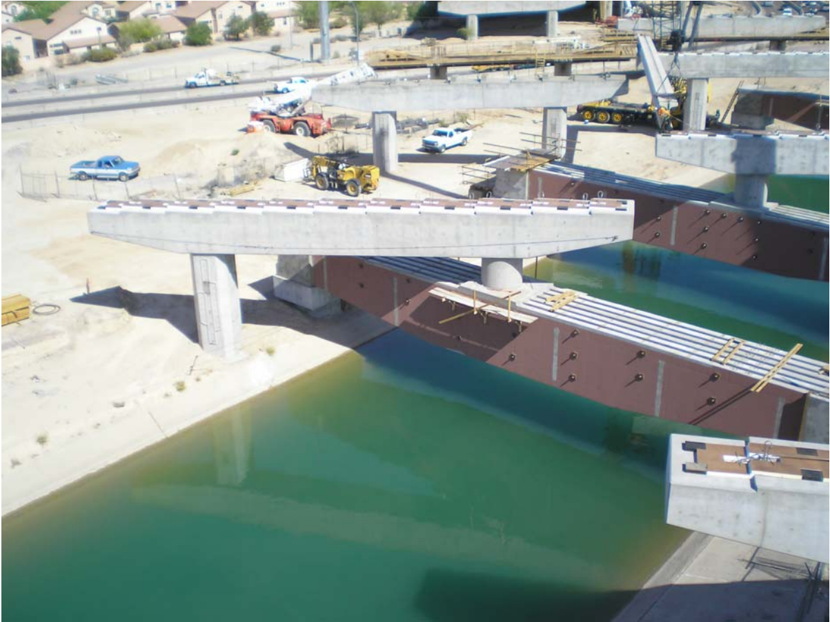
Fig. 9 – One of four straddle assemblies with stub column, full column, and cap beam.
