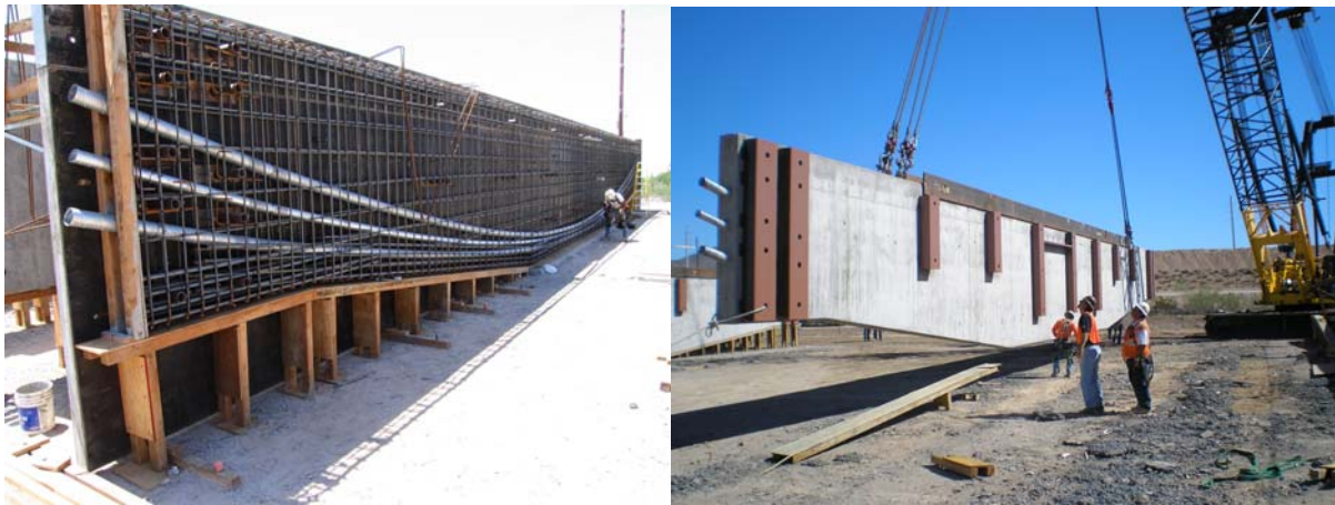
Fig. 10A – Precast ply during site production. Fig. 10B – Completed ply being erected.
