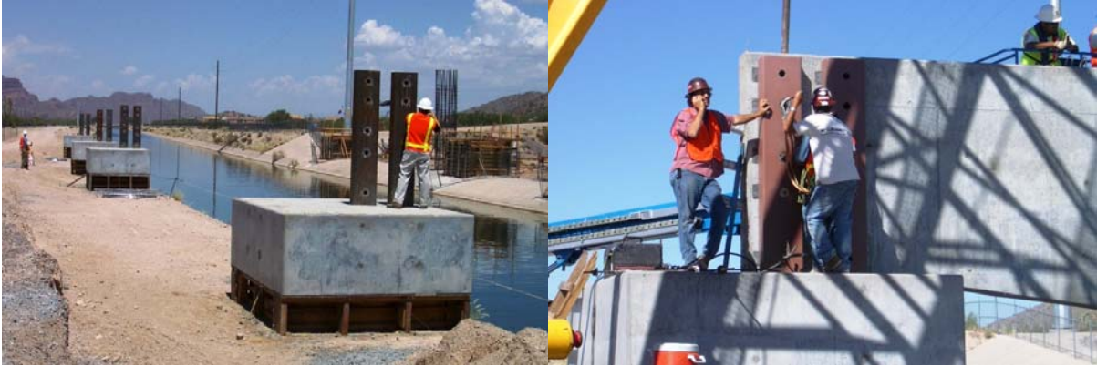
Fig. 12A – “Hitching posts” in drilled shaft caps. Fig. 12B – First ply is set.
