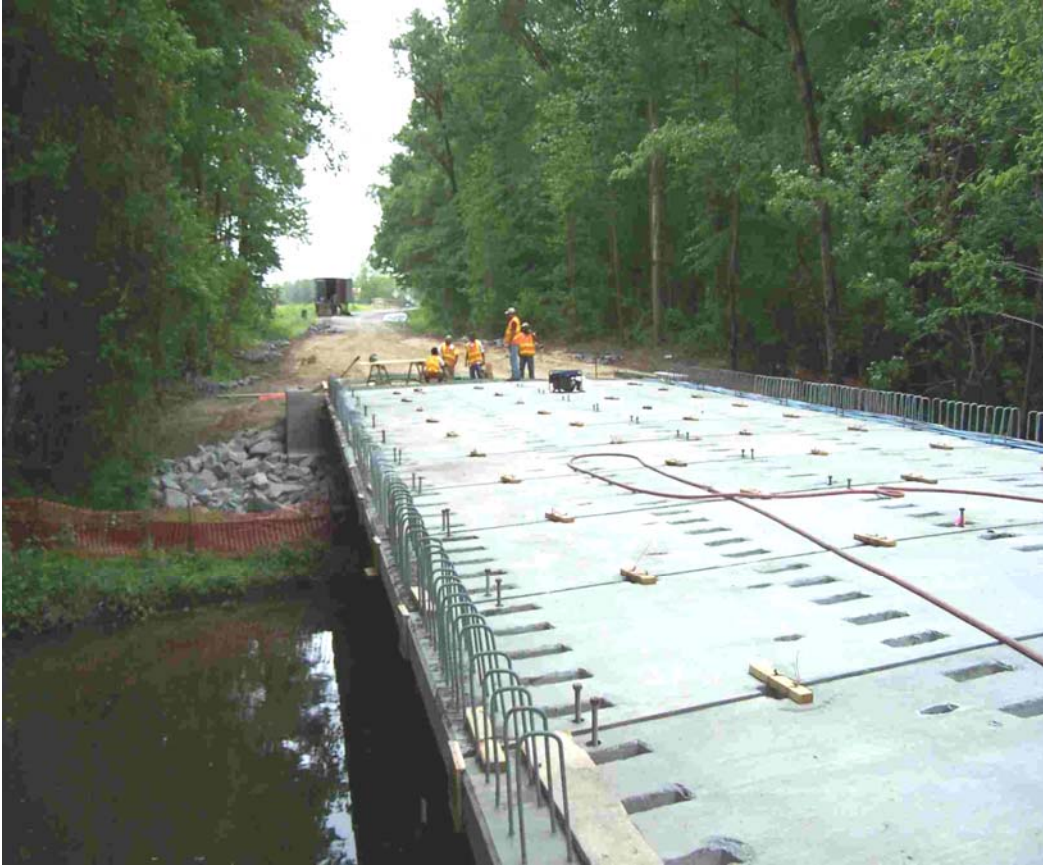
Figure 9 -- Once the transverse joints are grouted, the panels will be ready for tensioning
