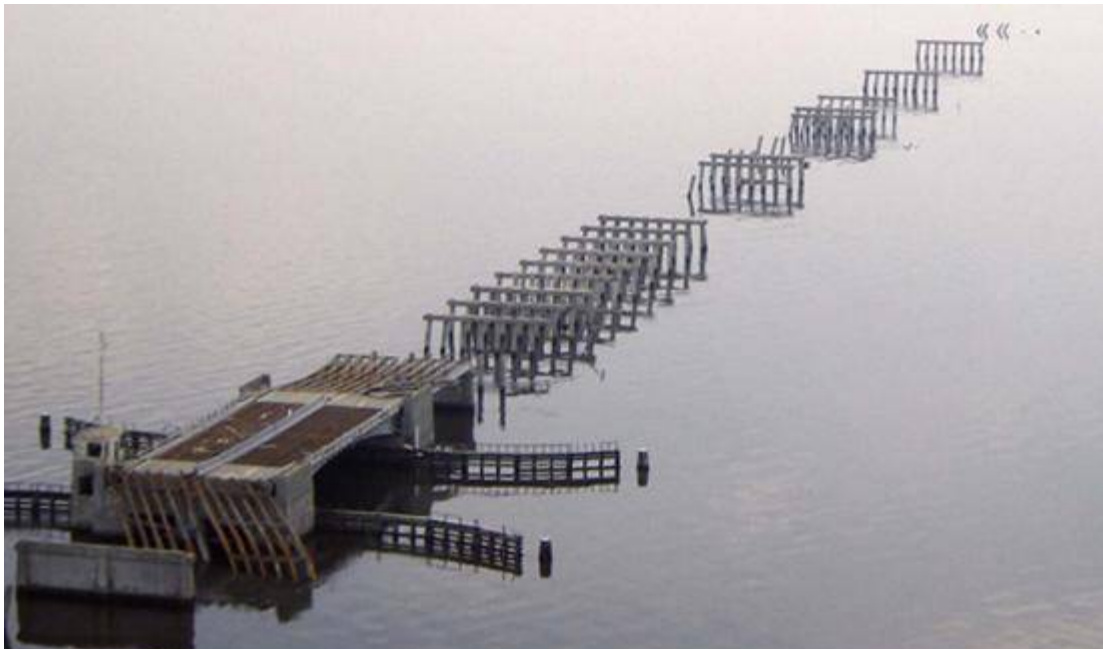
Fig. 1 Looking west from the destroyed Bay St. Louis Bridge bascule spans
