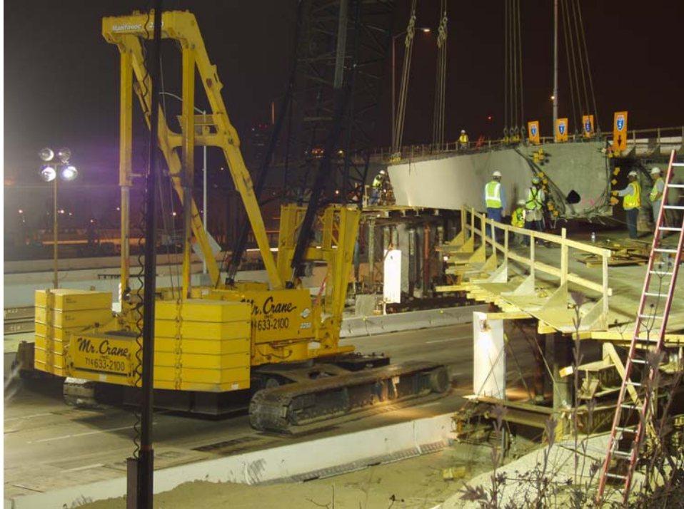
Fig. 7 A single crane lifts and transports the 240,000 lb girder from casting site to shoring supports.
