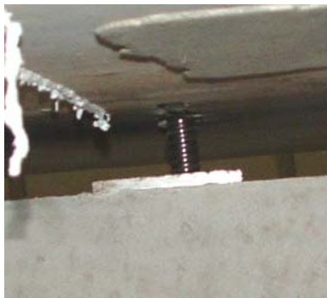
Figure 8 Leveling Bolt Bearing on a Steel Plate
