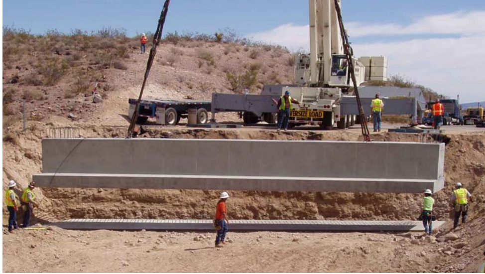
Fig. 2. Digital image portraying the placement of the precast abutment at the Marble Wash (Left) Bridge
