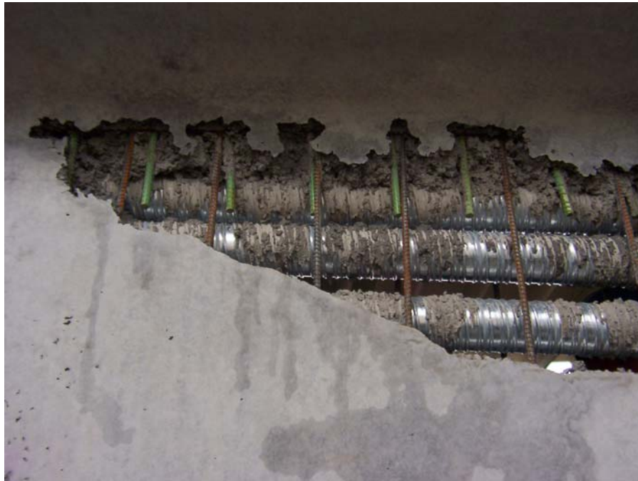
Figure 8 Typical void in the first few middle segments of girders produced
