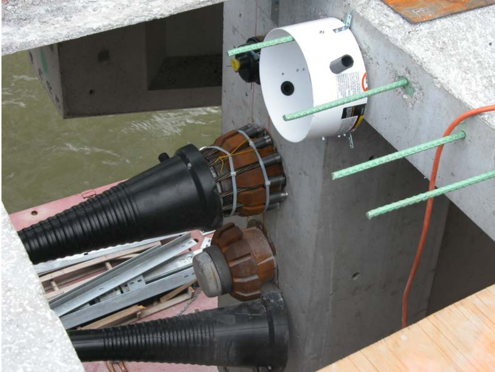
Fig. 4 Post-tensioning tendon couplers were utilized to provide continuous prestress in the longitudinal direction of the bridge and to prestress the cast-in-place splice joints. The plastic duct had to be modified to allow movement of the anchor casting during subsequent tendon stressing after the closure joint was placed. The duct modification was fabricated from plastic five gallon buckets.
