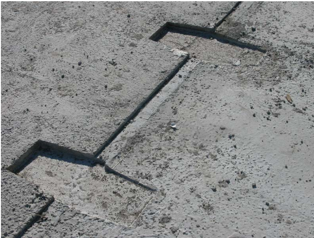
Fig. 2. The longitudinal slab joints and transverse post-tensioning tendon block outs are shown after filling with epoxy grout and concrete.
