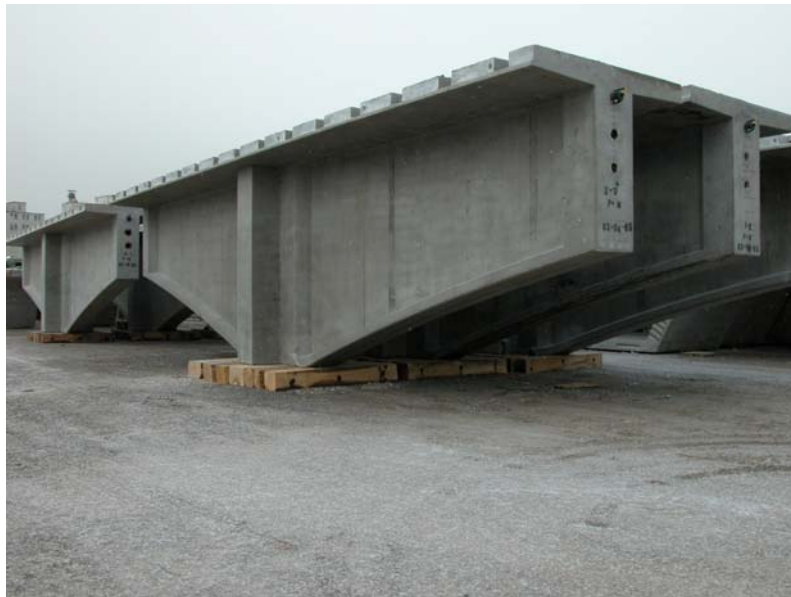
Fig. 5 Pier module segments were stored in the casting yard. The module in the fore ground with 03-04-05 casting date was the first module to be cast for the project. The top post-tensioning tendon is stressed in the form to carry the dead load handling stresses in the pier module.
