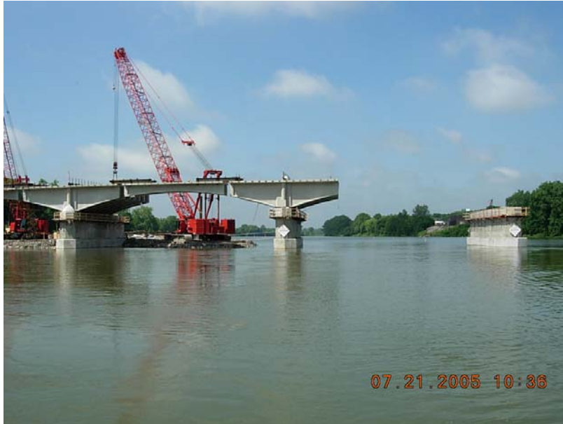
Fig. 8 The contractor chose to erect pier modules on piers 1, 2 & 3 in the first unit making the first post-tensioning tendons one span longer than was assumed in the design requiring no design changes but a shop drawing modification.
