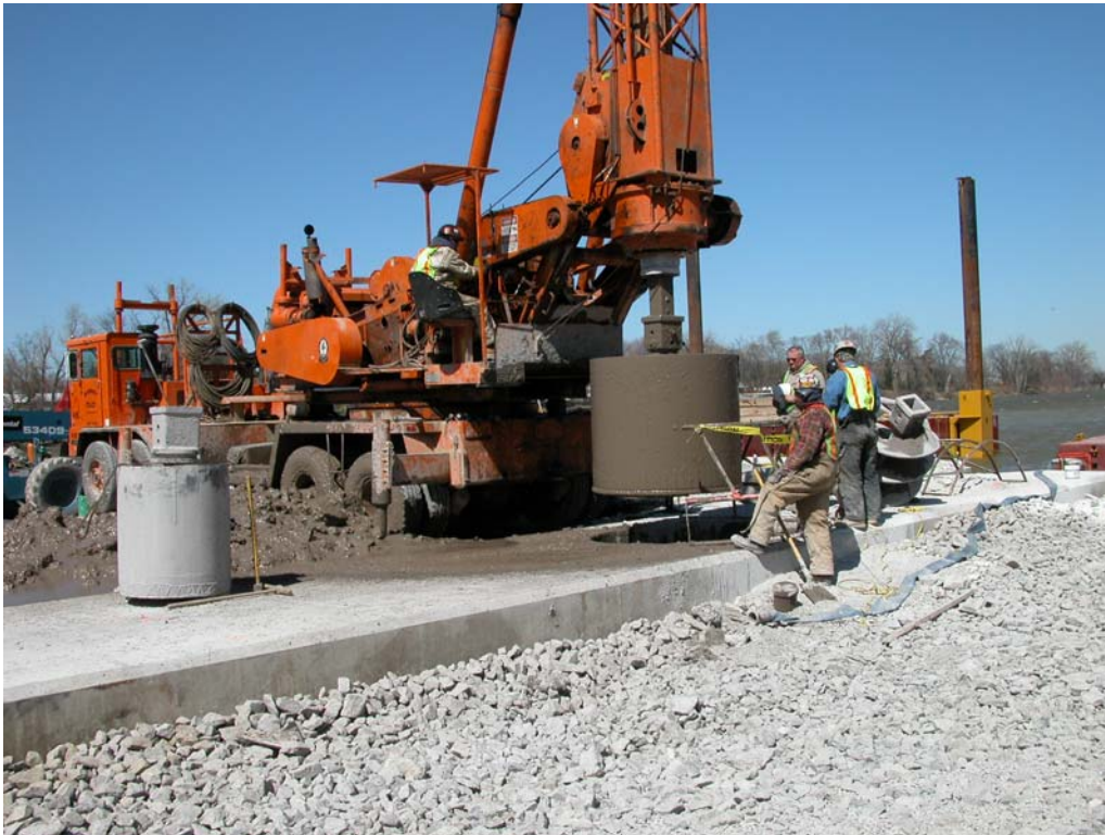
Fig. 3 Pilot holes, 42 in. in diameter, were drilled full depth through the leveling course and existing pier.
