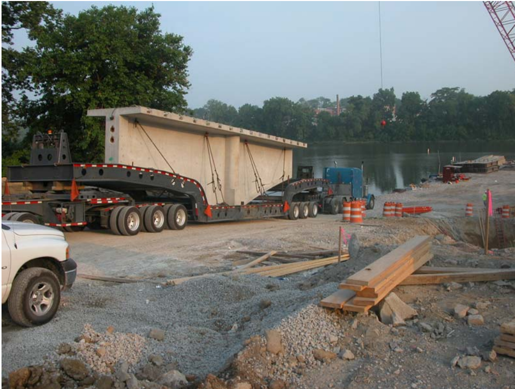
Fig. 7 The first module arrived at the site for erection on June 29, 2005. Special trailers were required to haul each of the different types of modules from the casting yard in Toledo to the construction site in Napoleon.
